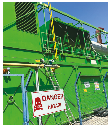
Gas Generator pipe inlet
