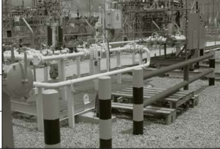
LEFT Over 2007 Orca increased the capacity of its low-pressure gas distribution system by adding a second pressure reduction station.
