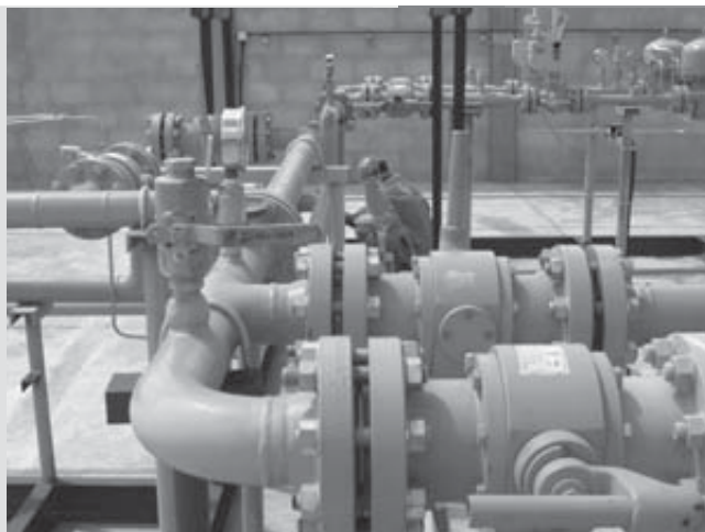
FAR LEFT: The new Wazo Hill cement plant kiln #4 is operating on Additional Gas supplied by Orca.
