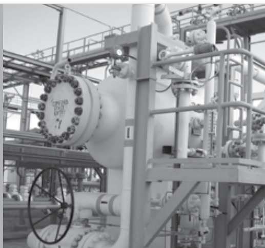
LEFT: Orca is participating in work to increase the capacity of the current gas processing and transmission infrastructure to 144 MMcfd.
